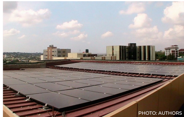
Figure 1: Solar PV installation at Consolidated Bank Ghana Ltd. (CBG), South Legon Branch by Tradeworks Co. Ltd.
