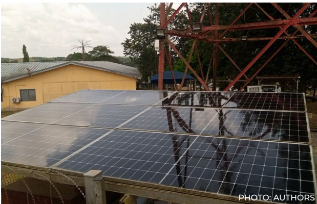
Figure 2: Solar PV installation at the Dabase site, operated by Helios Towers
